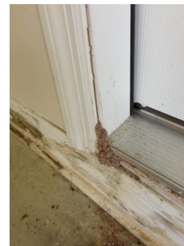
Fig 2. Mud tube and trim separation from door frame
