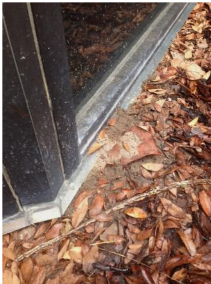
Fig 3. Exterior door frame creating a structural joint along the foundation of the structure. Photo by M. Bentley, University of Florida
