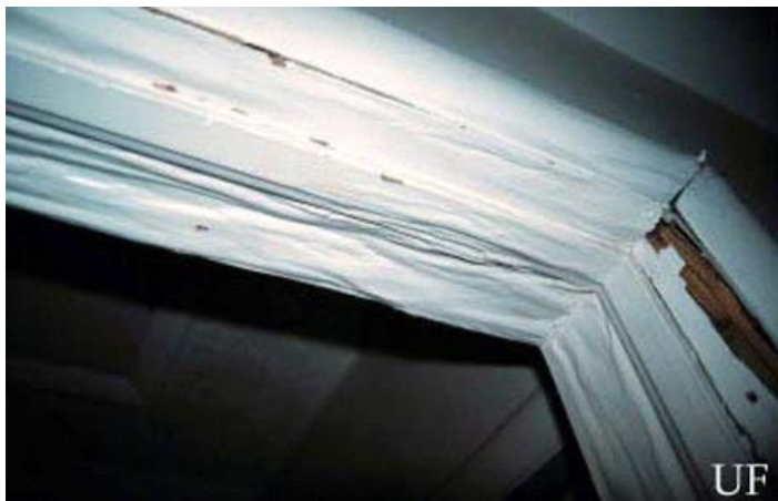
Fig 6. Termite damage to door frame. Photo Credit: http://entnemdept.ufl.edu/creatures/urban/termites/formosan_termite.htm
