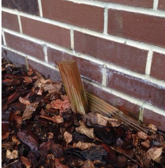
Fig 5. Stray cellulose left along the foundation of a structure. Photo by M. Bentley, University of Florida
