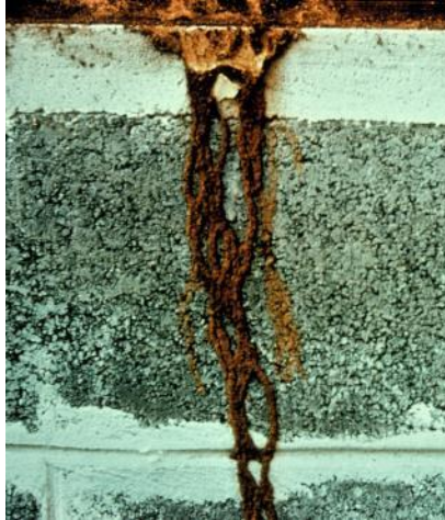
Fig 2. Termite mud tubes at the foundation of a home. Photo by J. Castner, University of Florida.
