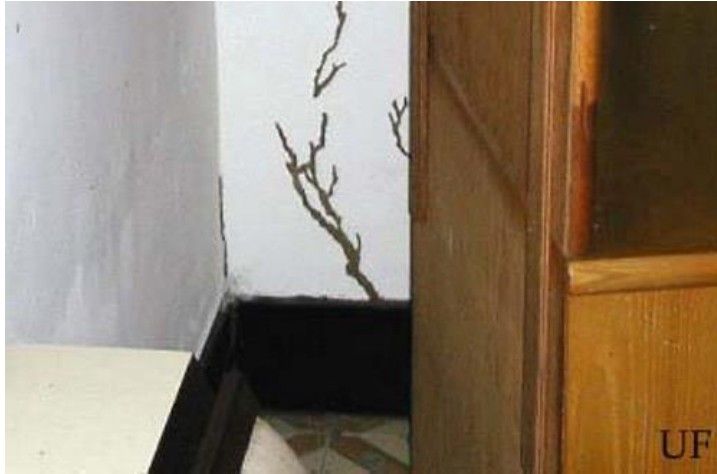
Fig 7. Termite mud tubes located behind a book case. Photo Credit: http://entnemdept.ufl.edu/creatures/urban/termites/formosan_termite.htm
