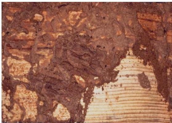
Fig 2. Eastern subterranean termite damage. Photo: J. Castner, UF.
