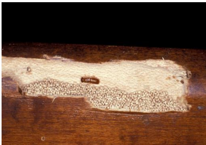
Fig 6. Drywood termite damage, fecal pellets, and alate. Photo: J. Castner, UF.
